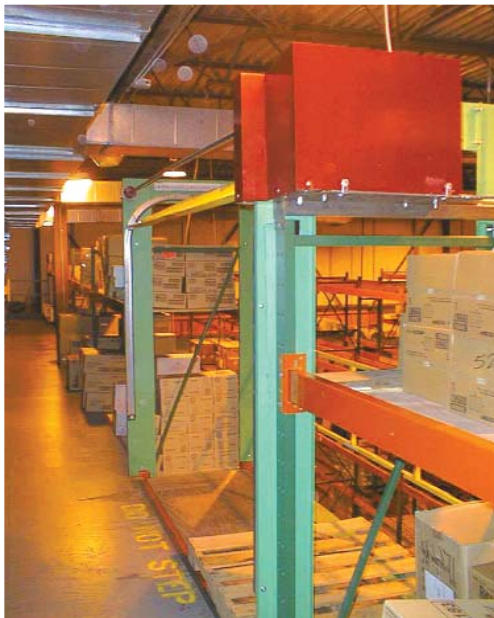
A Rack Supported Safety Gate in Grocery Supply Company's Sulphur Springs facility.
